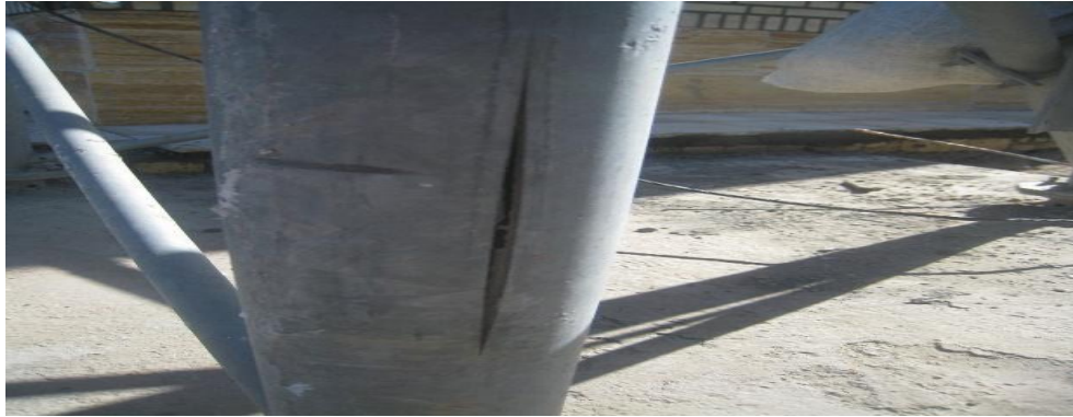
Fig. 5. Tear of the base of TV & FM tower due to lightning strike.
