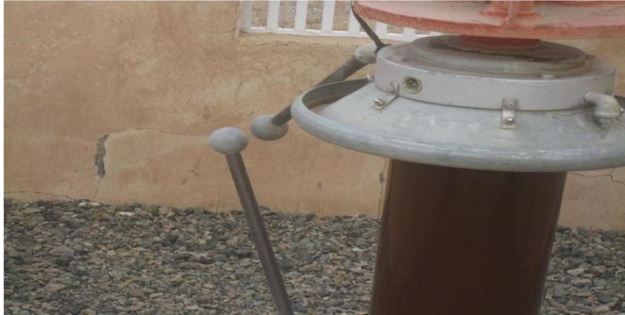
Fig. 9. Superficial demolition due to lightning strikes.
